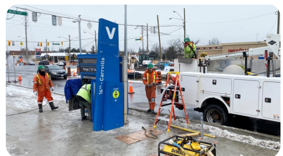
Vivastation identification "fin" in place
