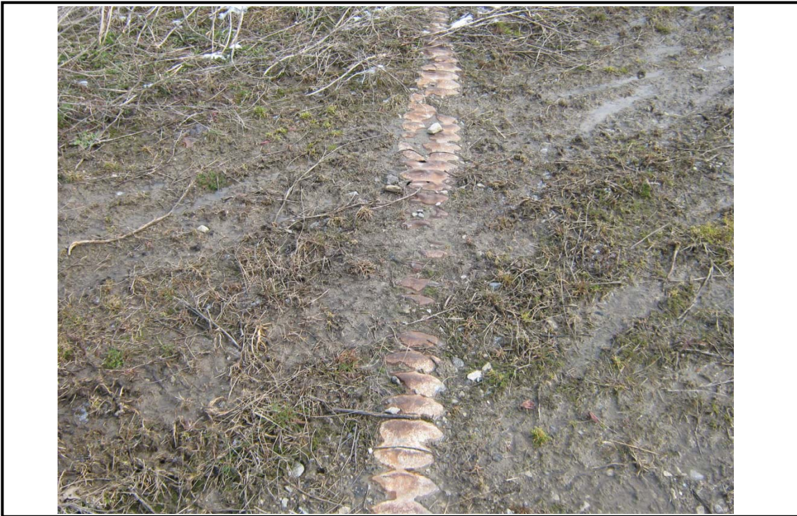
Photograph 7: Corrugated steel pipe that appears to be used for stormwater management directing the stormwater to the Site perimeters.
