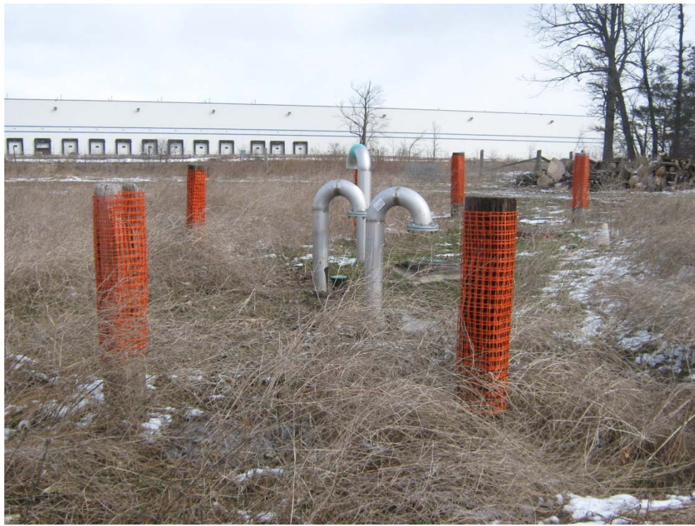
Photograph 3: View of the Black Creek pump station located on the northern portion of the Site (west of the wooded area).
