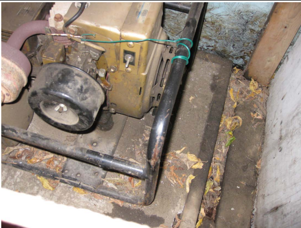
Photograph 6: View of the generator at Rocco Farms.
