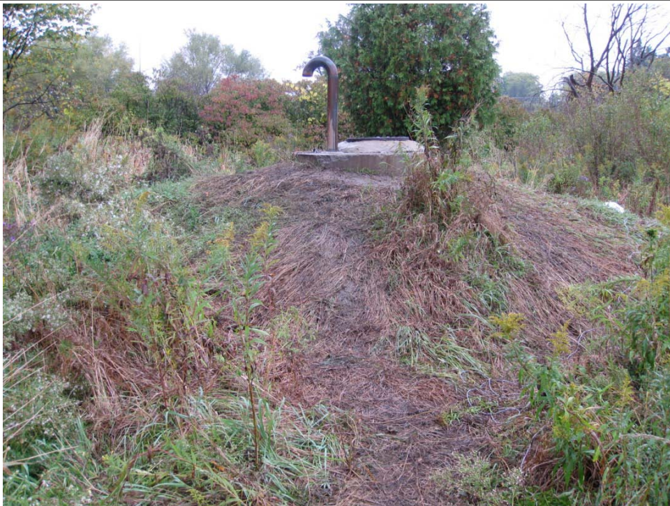
Photograph 17: View of what appears to be a sanitary connection and a vent pipe observed on the southeast area of the Site.
