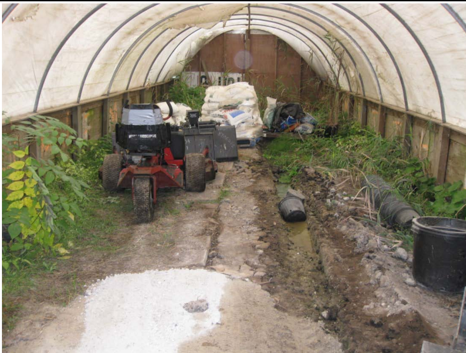
Photograph 23: View inside the greenhouse structure observed in the area occupied by Nino's Landscaping.
