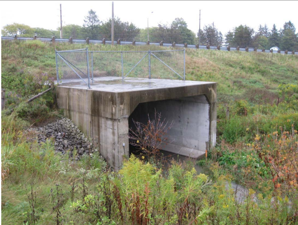
Photograph 1: View of the culvert for Black Creek located on the east Site boundary.
