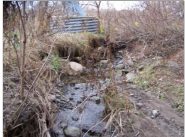
Reach 11 – Tributary 1 downstream of Jane Street, eroding banks
