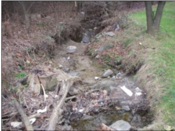
Reach 10 – upstream of Jane Street at cemetery, Eroding banks
