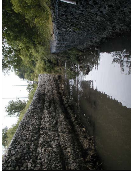
Photo 6: Dufferin Creek crossing at Dufferin Street facing upstream (south) from the culvert.
