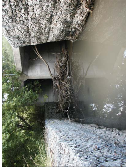
Photo 7: Dufferin Creek crossing at Dufferin Street facing downstream (north) towards the culvert.
