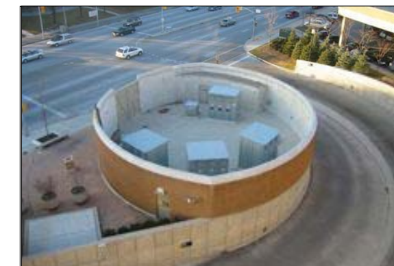
Electrical Substation (Don Mills Station)
