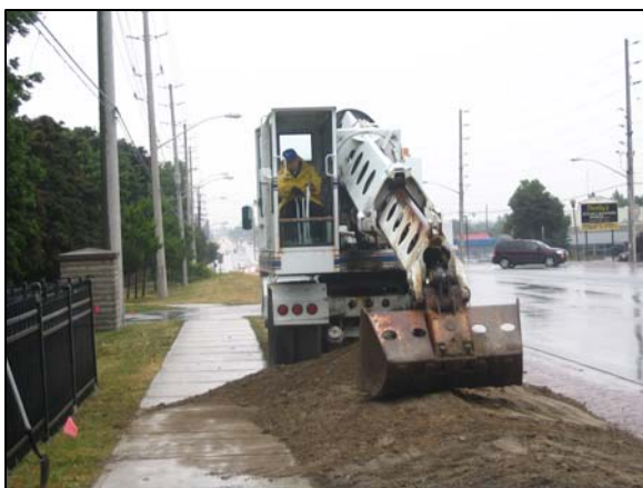
Plate 5: Looking north at the Gradall operator backfilling a trench segment to its original grade.
