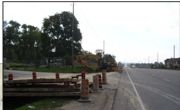
Plate 6: View to south along Yonge Street from entrance to Summit Golf Club. ROW has been previously disturbed. Potential may exist beyond fence line.
