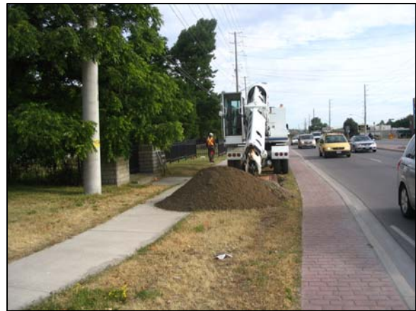
Plate 4: Looking north at the Gradall excavation between the sidewalk and the curb.
